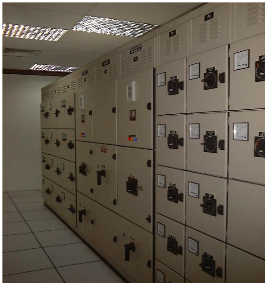
Main Switch Board
